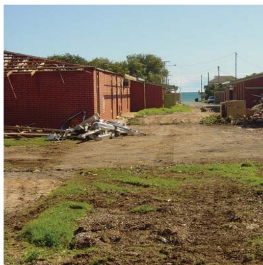
The old school buildings are reduced to rubble and amazing sea views have appeared for the future site of Townsend Park - Stage Three.
